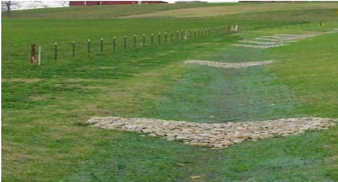
Plate 5.3: Photograph of Check Dams
